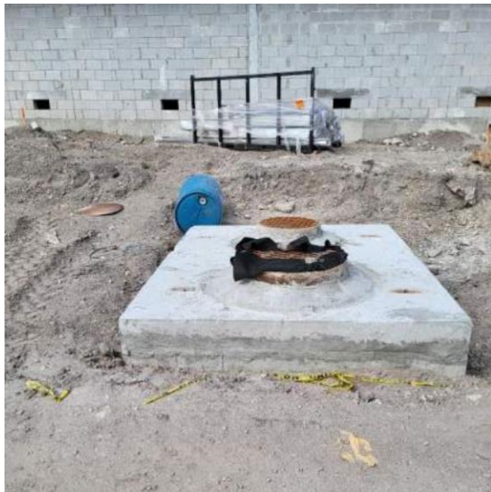
Fig. 1. Installed drainage well structure observed during the mid-construction stage, showing that stormwater infrastructure was already materially in place before final grading and site stabilization were completed.
