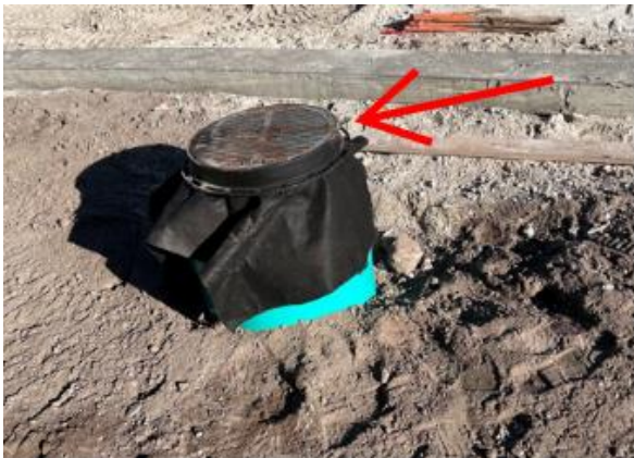
Fig. 7. Reinstated temporary covering at Yard Drain 6 after the reported deficiency, showing immediate field protection used to interrupt further sediment entry into an active drainage feature.
