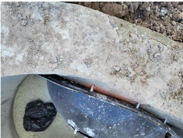
Fig. 5. Questioned baffle installation at MH-21, showing a vulnerable internal control detail with visible gap and questionable fastening condition.
