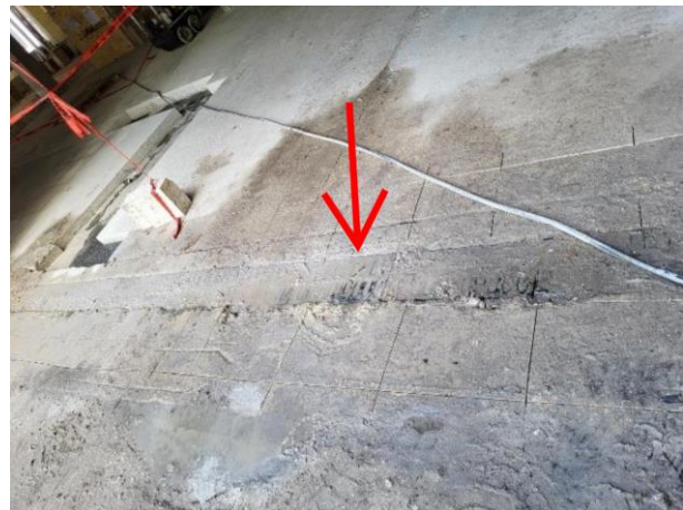
Fig. 6. Sediment-filled trench drain at the existing driveway interface, illustrating localized loss of drainage collection capacity during active construction.
