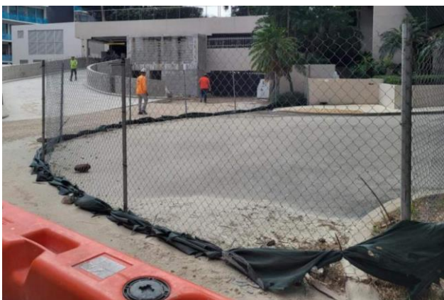
Fig. 2. Temporary sediment-control measures requiring maintenance, with sediment tracking visible outside the
