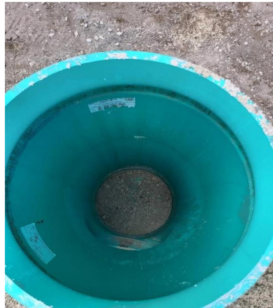
Fig. 4. Sediment observed inside Yard Drain 6, showing progression from exposure risk to actual intrusion at an active collection feature.
