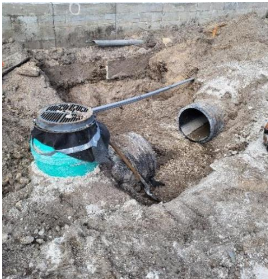
Fig. 3. Exposed Yard Drain 10 during lateral fitting work, showing a live drainage intake and connected piping temporarily left vulnerable to sediment intrusion.
